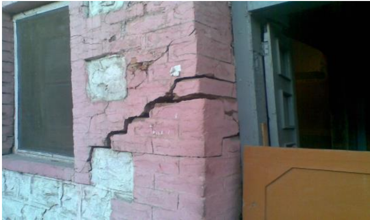
Fig. 3: Large crack in the wall
